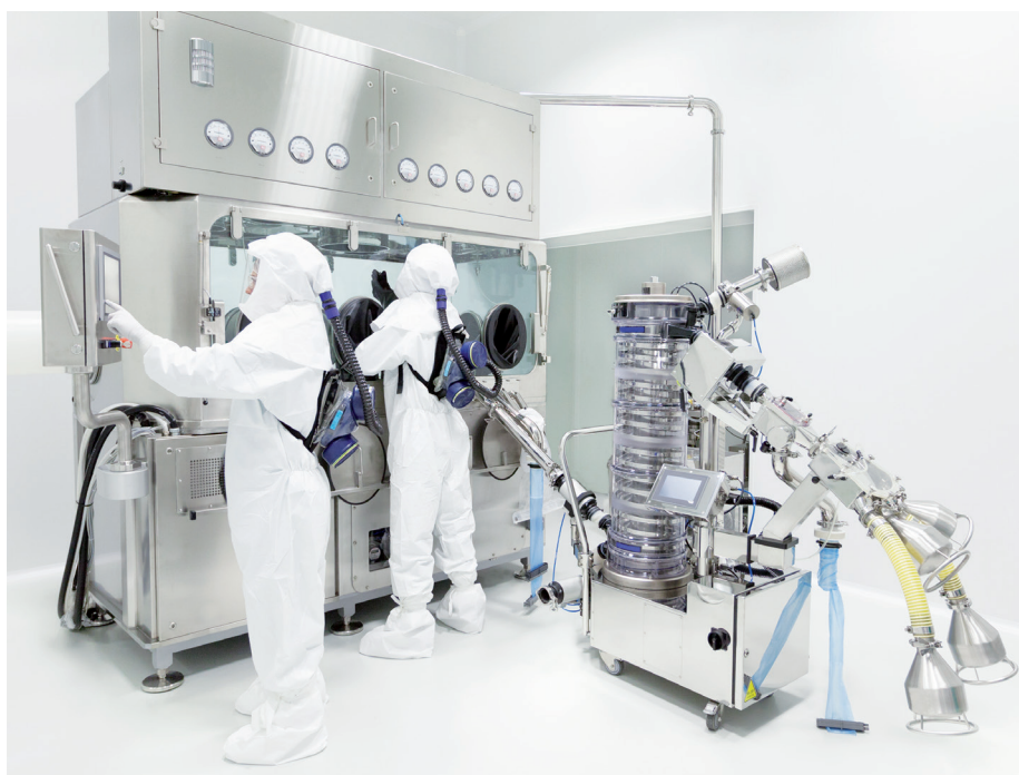
Figure 1: Large-scale capsule filling process at one of Hovione's manufacturing lines.
